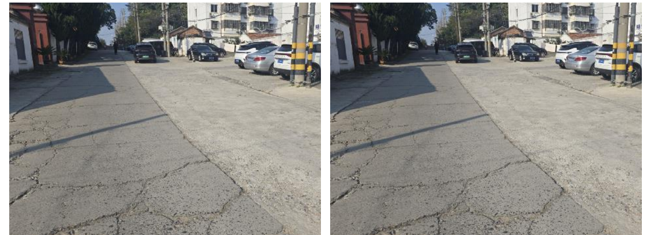
破碎板及纵向裂缝
